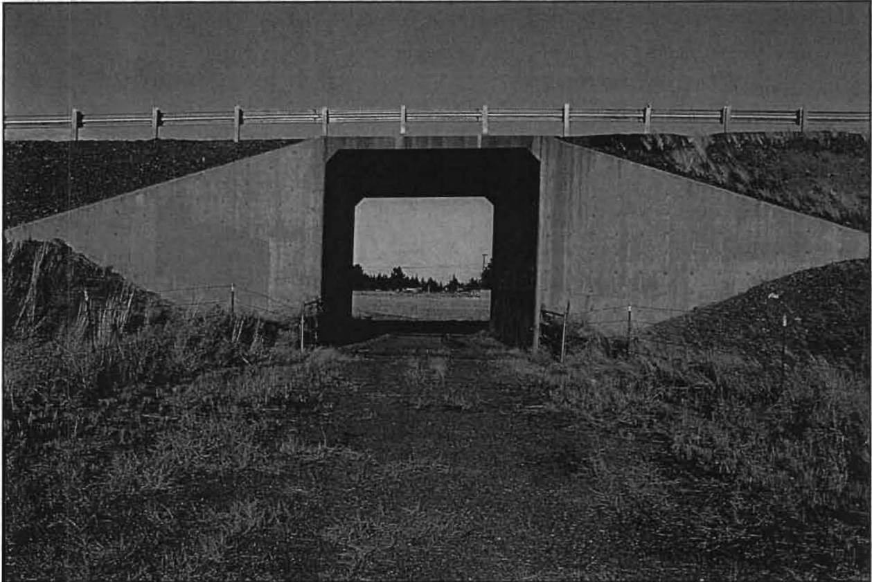
Small 16' box culvert built to allow internal road across the Aceti-Barrett private property on the west side of US Highway 97 as part of mitigation for the Deschutes Junction Overpass project. Photo repeated from Application
