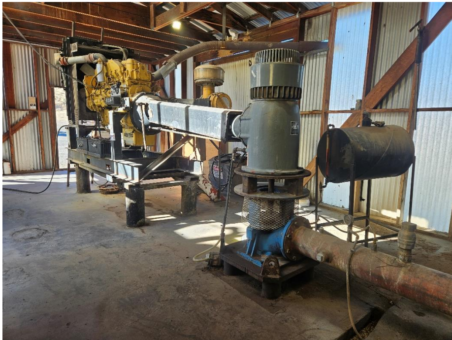
Photo 2. The interior of the active well (Well B) house, as seen from the northeast.
